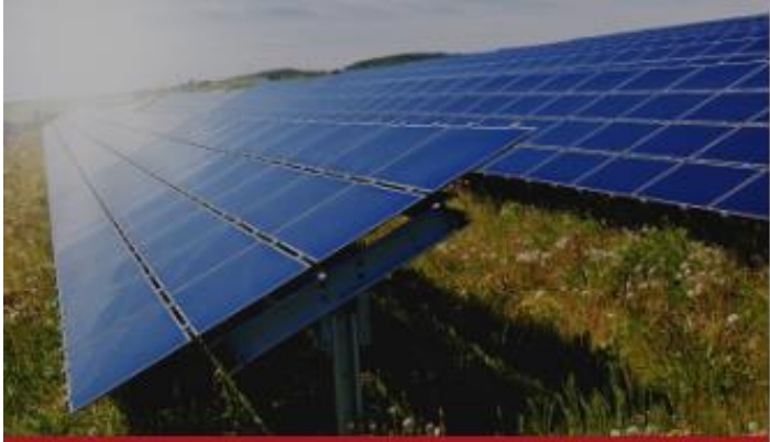
10kW Solar Demonstration
